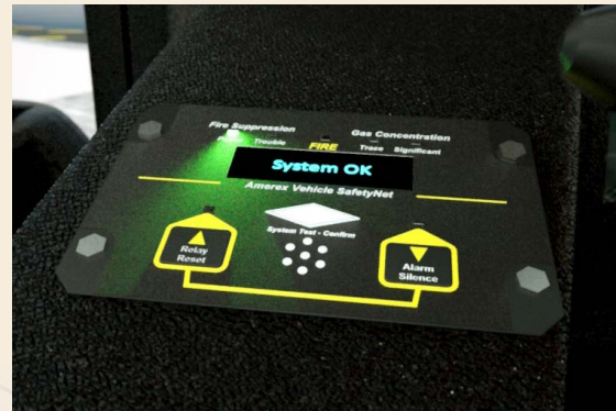
SafetyNet Display Panel
